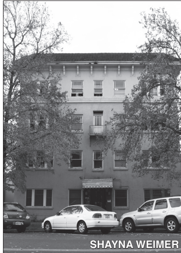
SHAYNA WEIMER Costs to renovate Haseldorf exceed how much money it would take to rebuild the apartments.
