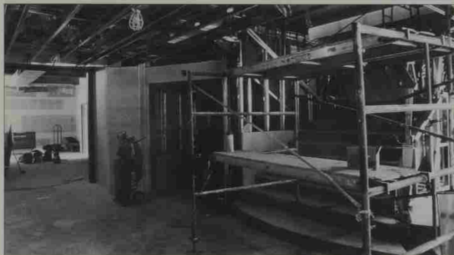
The construction crews at the Museum of Art were hard at work this spring, preparing for a fall opening.
