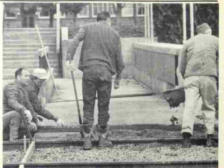
With nearly two month's of usage the newest crossing of the millstream was out of use during the middle of the week to allow fresh concrete to set.
