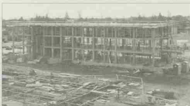
LEFT: Kaneko Commons is scheduled to open fall 2006. ABOVE: The atrium and dining facility will still be under construction until Jan. 2007.
