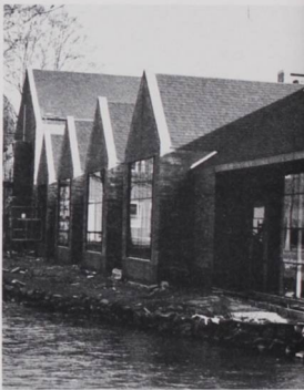
Once construction got started on the outside of the dining commons it moved right along.
