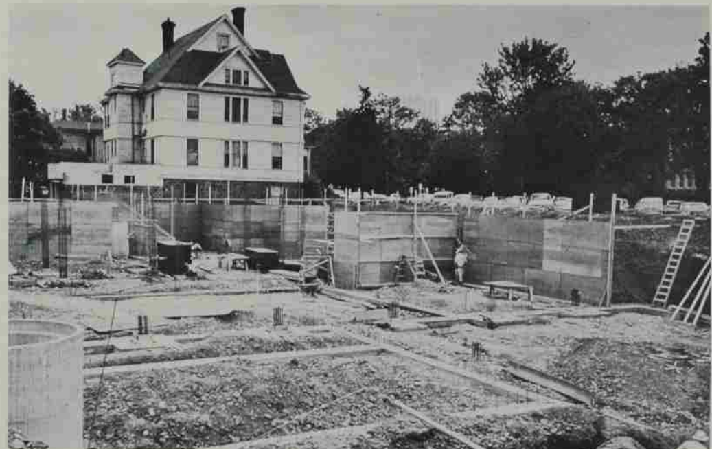
. . . and this is what came of it. The Truman Wesley Collins Legal Center will rise here, a memorial to the father of the youthful ground breakers. (Old building in background will be removed.)
