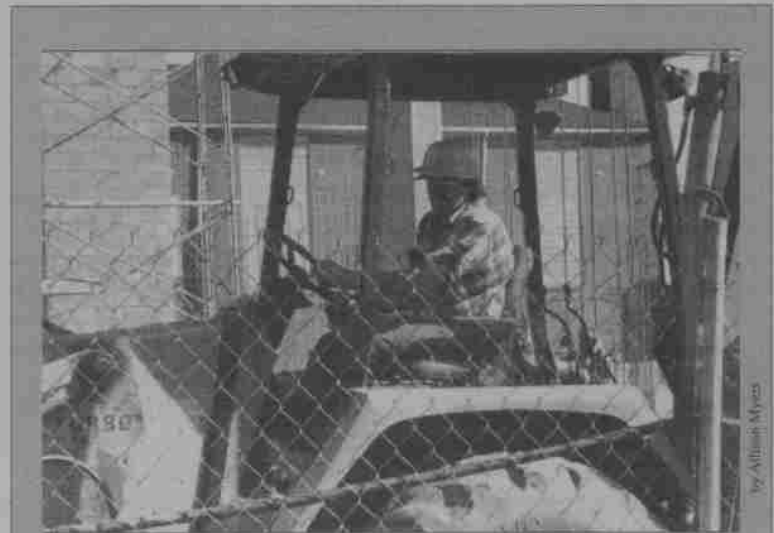
Sean Donne uses the bulldozer to clear away gravel during the ongoing construction of the music building.
