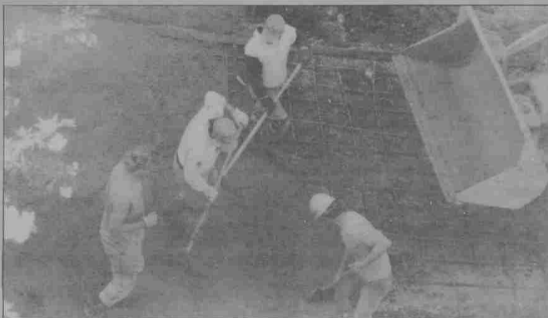
Four construction workers at the Olin Science Center construction site smooth the cement poured for a walkway which will circumscribe the future building. A clear day allowed the workers to pour the cement and a small team spent much of Wednesday smoothing the surface of what will be Willamette's newest student byway.
