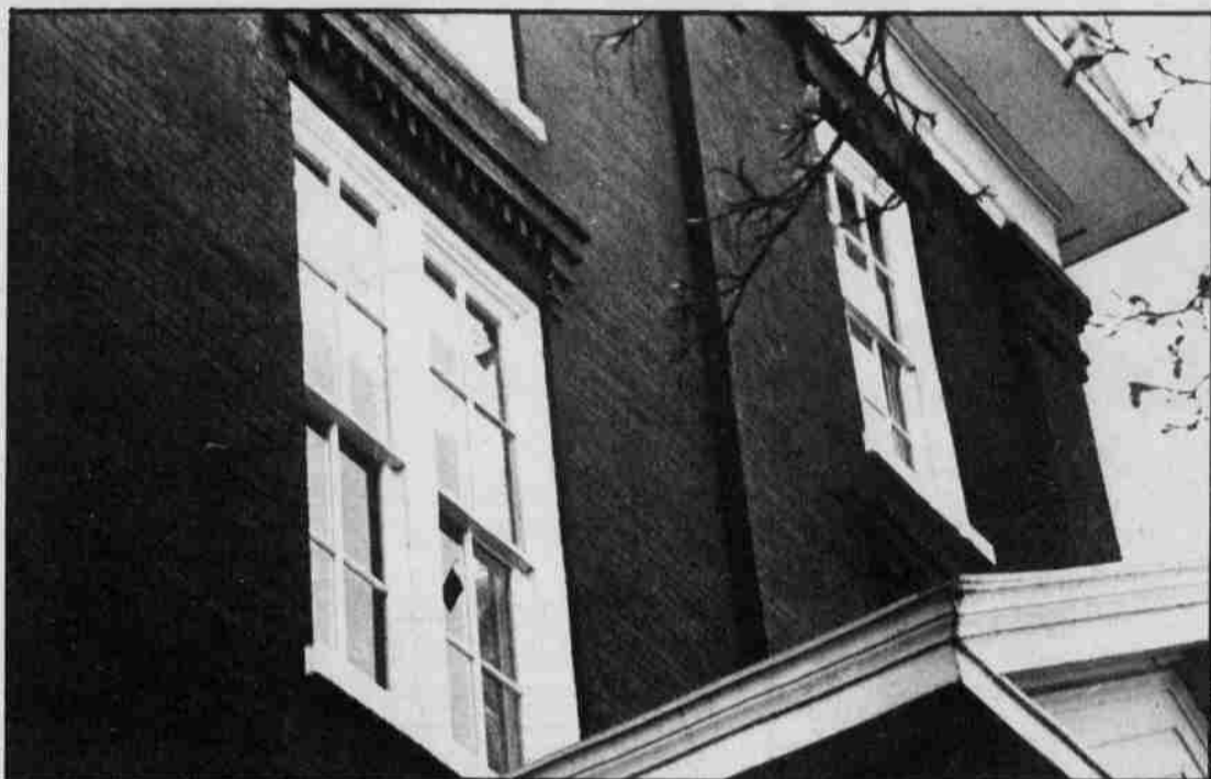
Thirty-four windows were broken in Waller Hall as a result of the quake.
