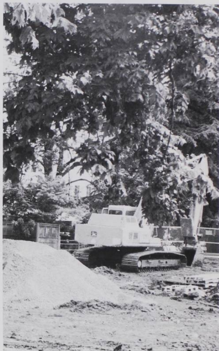
Piles of dirt occupy the former grounds of the University House as construction begins on the Olin Science Building.
