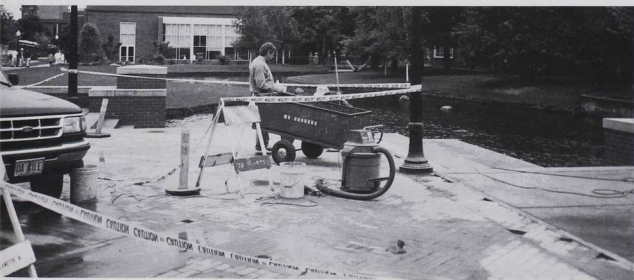
Bricklayers work at a feverous pace to replace broken bricks in Jackson Plaza by graduation.
