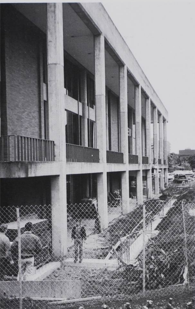
Deep trenches occupy the space where the U.C. stairs used to be paving the way for new construction.
