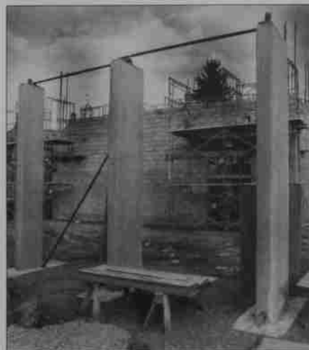
The newest building on campus rises from the former Bishop Health Center site. This music center and recital hall is expected to open spring semester, 1998-99.
