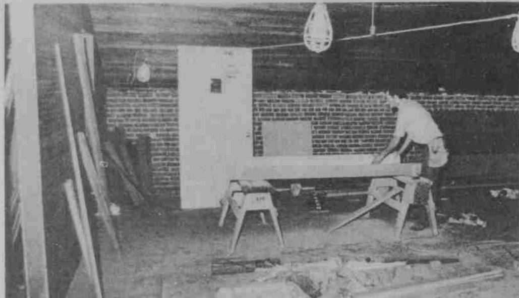
A lone construction worker begins the arduous task of remodeling the Art Building.
