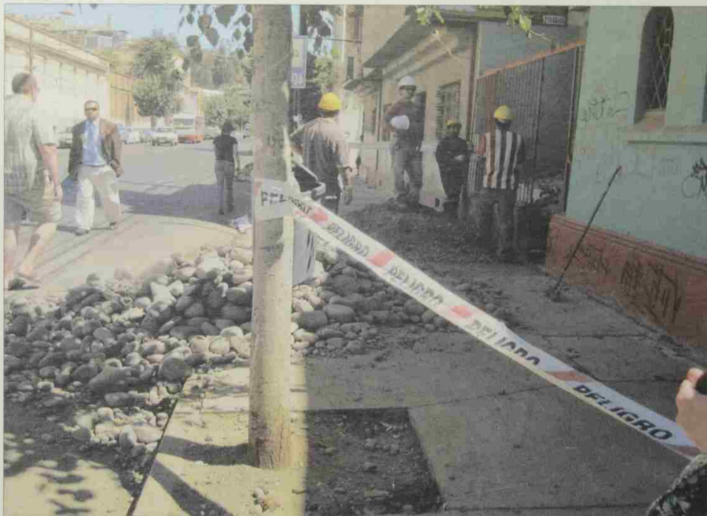
Damage on the city street in capital Valparaíso.
