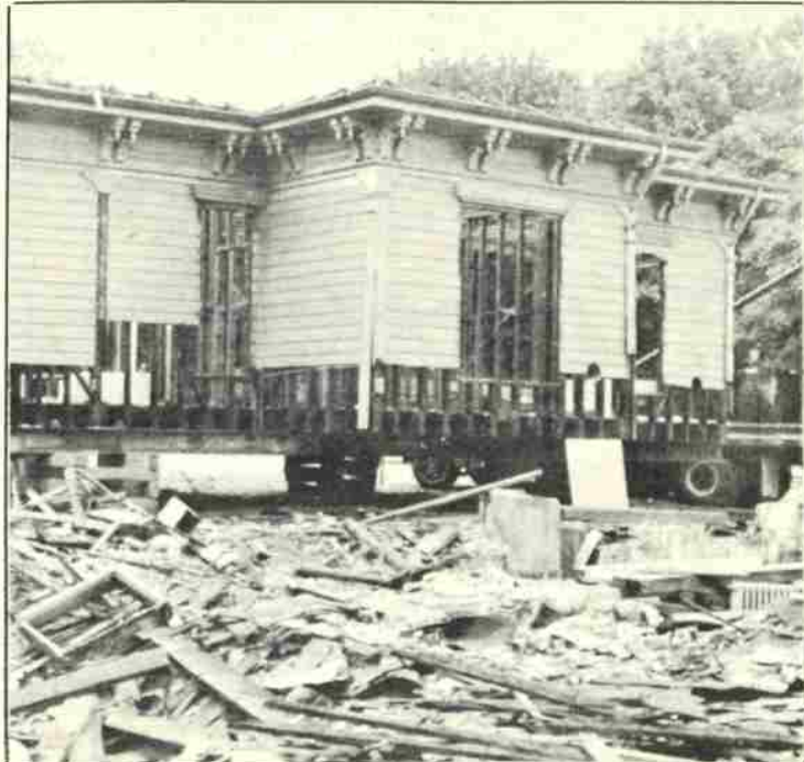
The 87 year-old Port-Manning house (across from Lausanne) is finally being dismantled and sent to its final resting place. (photo by Walker)
