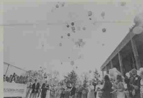
Top: Senators Packwood and Hatfield converse at April 13 groundbreaking; library site is directly behind them. Left: Sen. Hatfield is flanked by President Jerry Hudson (left) and Sen. Packwood as he hoists the first shovelful of earth; release of balloons marks the moment.
