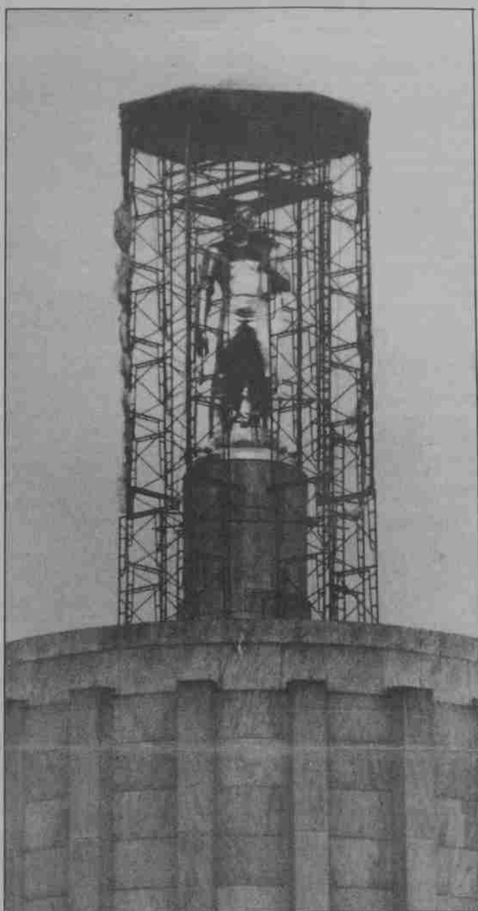
The Pioneer shown in a web of scaffolding has been re-coated, and now shines unobstructed over the Capitol City.
